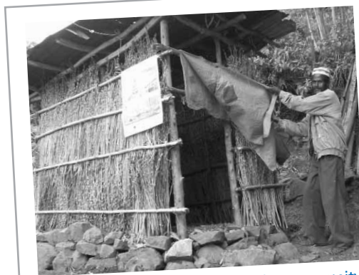
2. Constructed by a member of the community's water management team, this latrine serves as a model for other community members.
